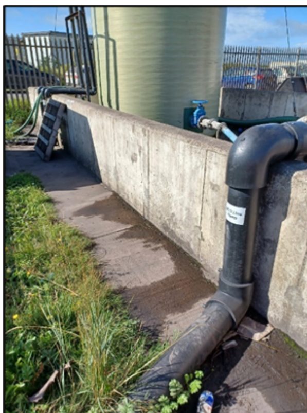
Figure 3 - Potential seepage through bund wall
