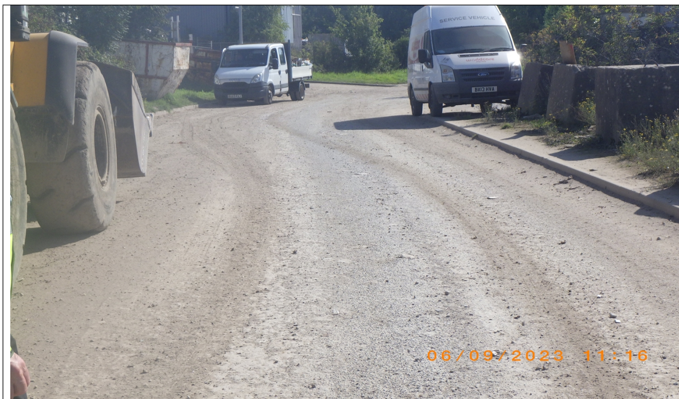
Photograph showing dust emissions to air and mud and debris on the highway.
