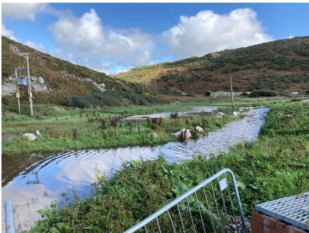
Flooding at the back of the beach caused by outfall blockage.
