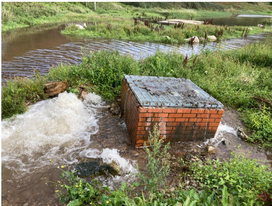
Flooding at manhole caused by outfall blockage.
