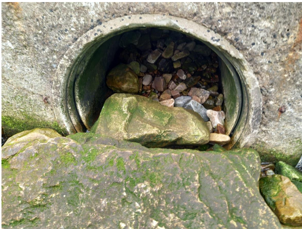
Substrate blocking outfall opening (b)
