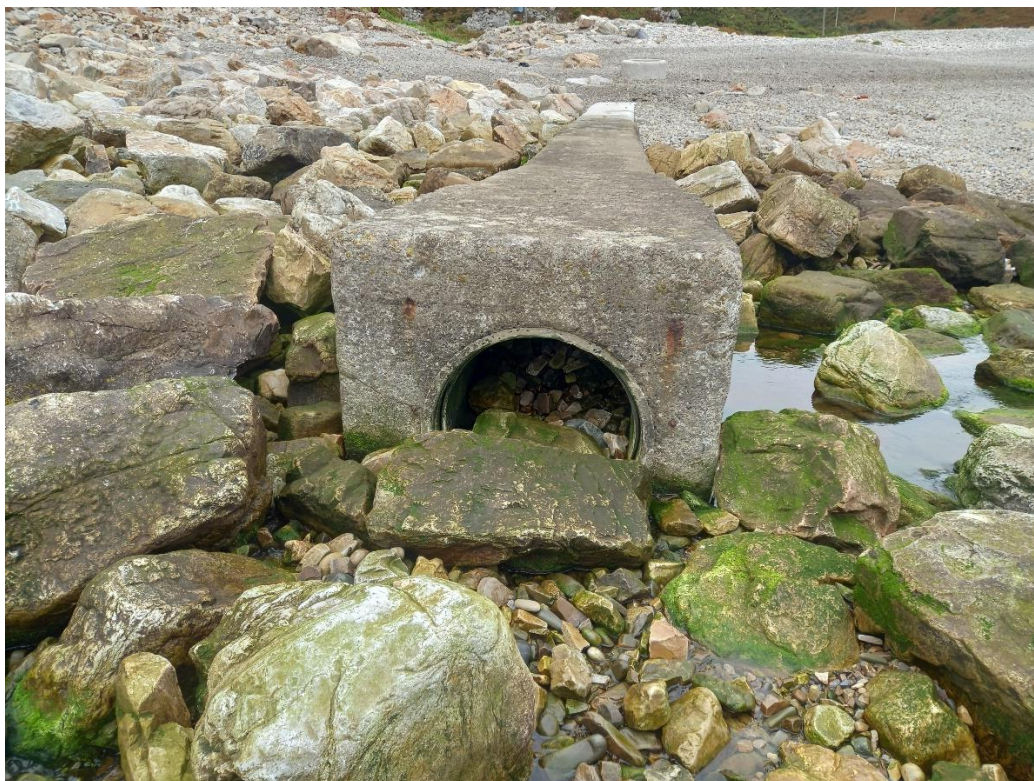
Substrate blocking outfall opening (a)
