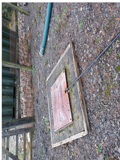
Photo 2 (Current system, Chamber/Cess Pit)
