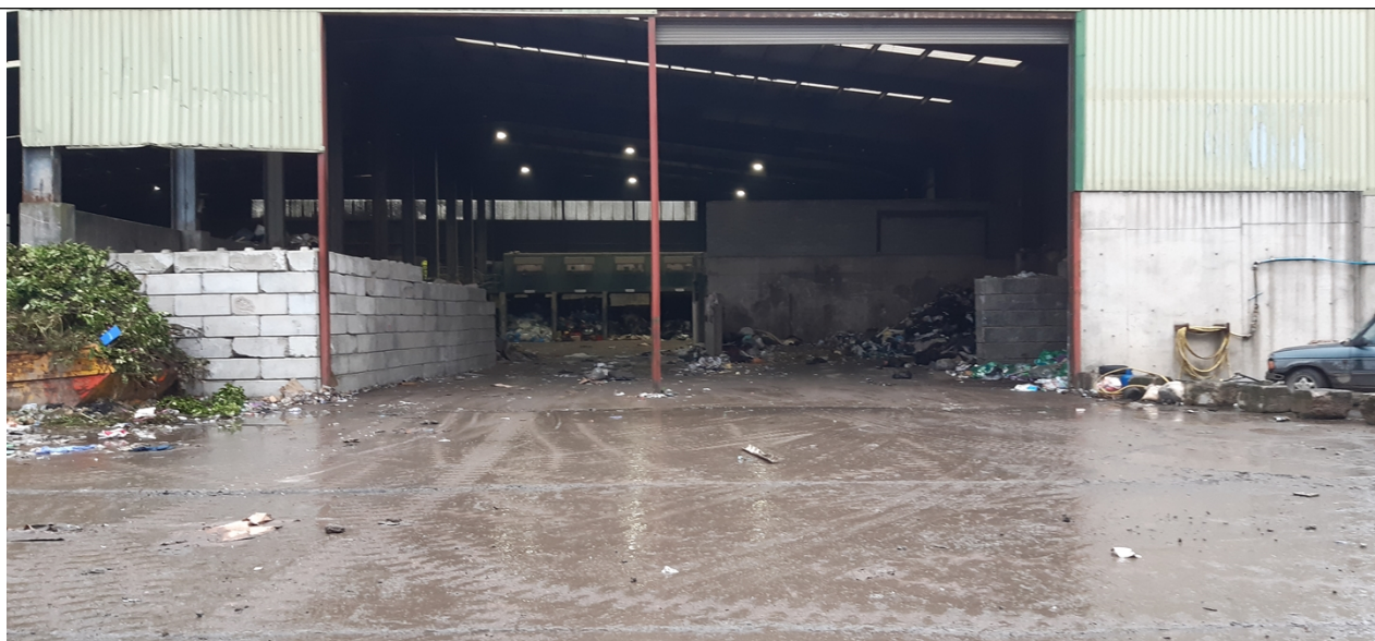
Photo 3 - View inside waste transfer station building
