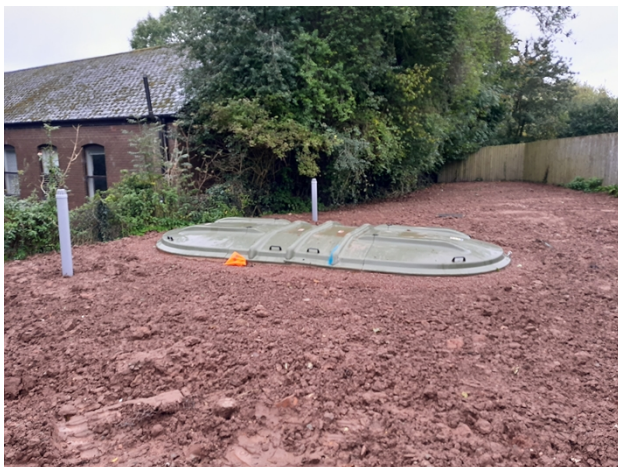
Effluent storage tank
