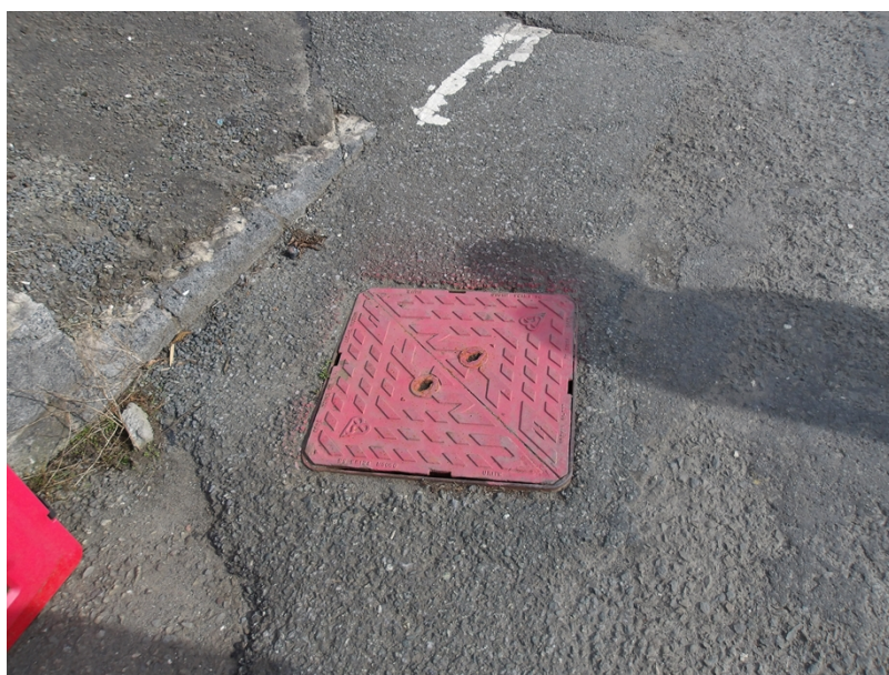
LTT/1 - Drainage covers colour coded
