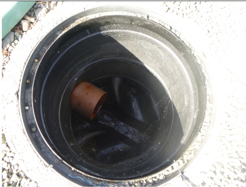
Photograph 2: Final effluent sampling point
