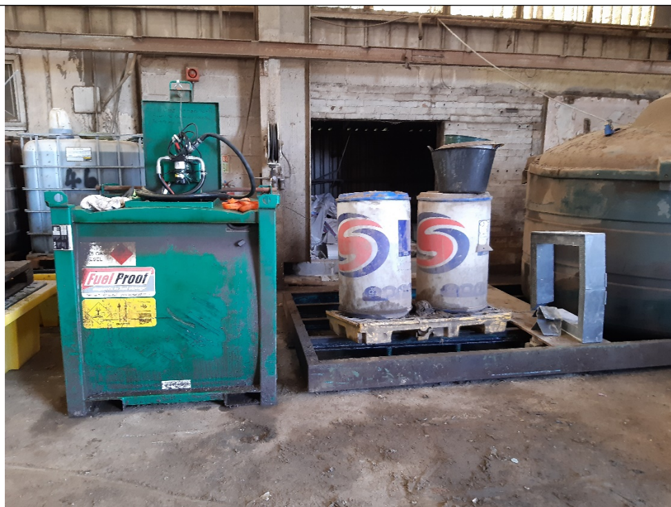
Photo 6 – bundled trays with IBCs within Unit 6 and other chemicals placed on them.
