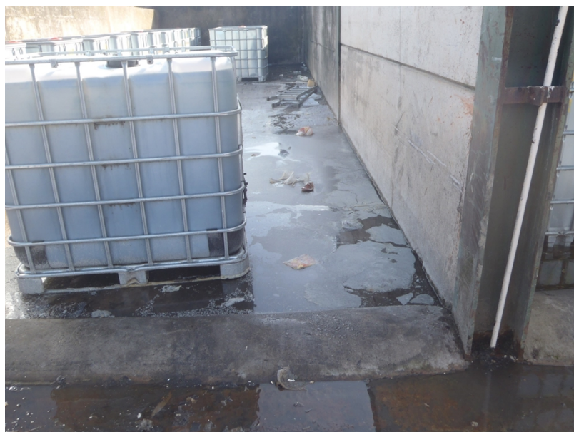
Liquid in bunded area
