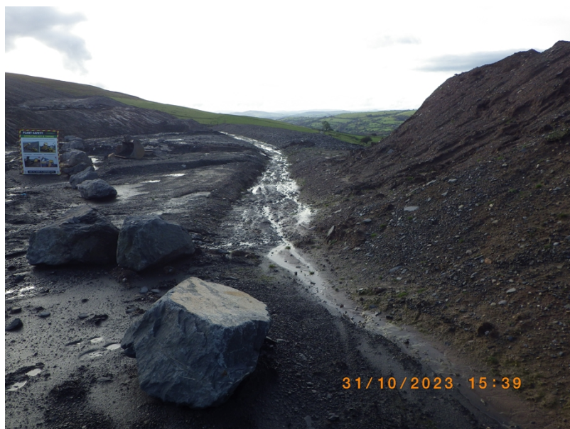
Surface water channel
