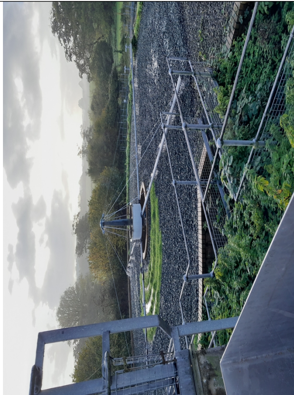
Grass and ponding visible on the filter bed
