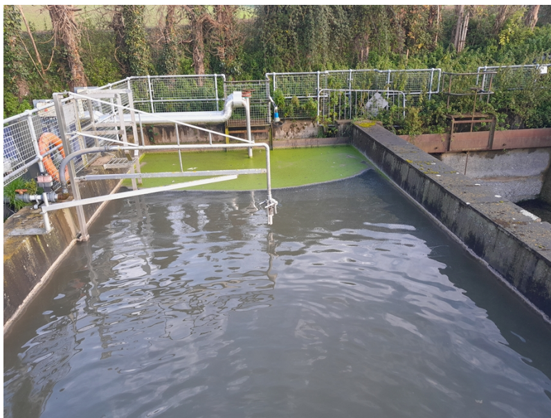
Storm tanks filling
