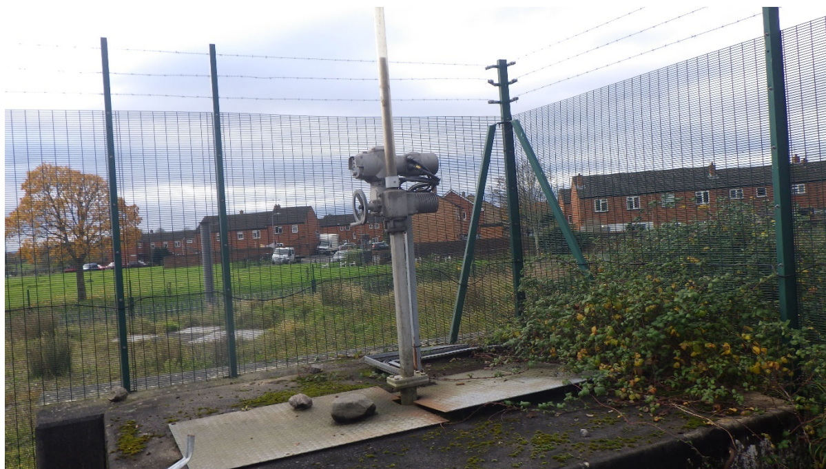
Figure 7: Site visit photos – Final penstock before storm line leaves site. Condition of the chamber covers is noted as a general improvement consideration.
