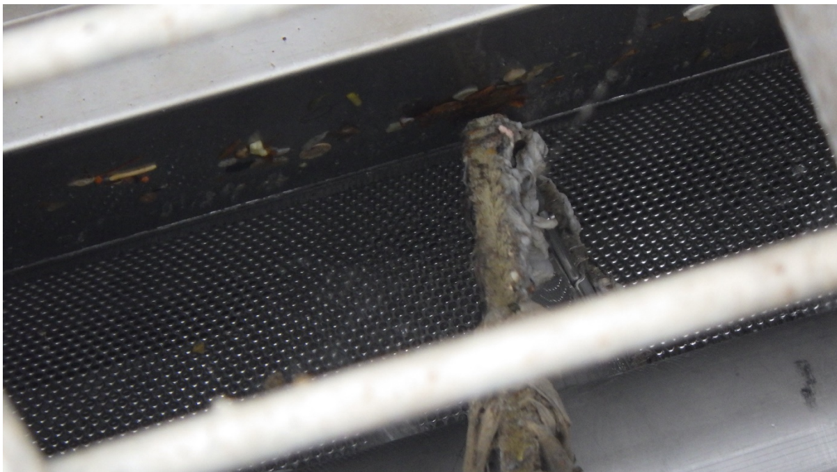
Figure 4: Site visit photo – screen condition at the time of the visit.
