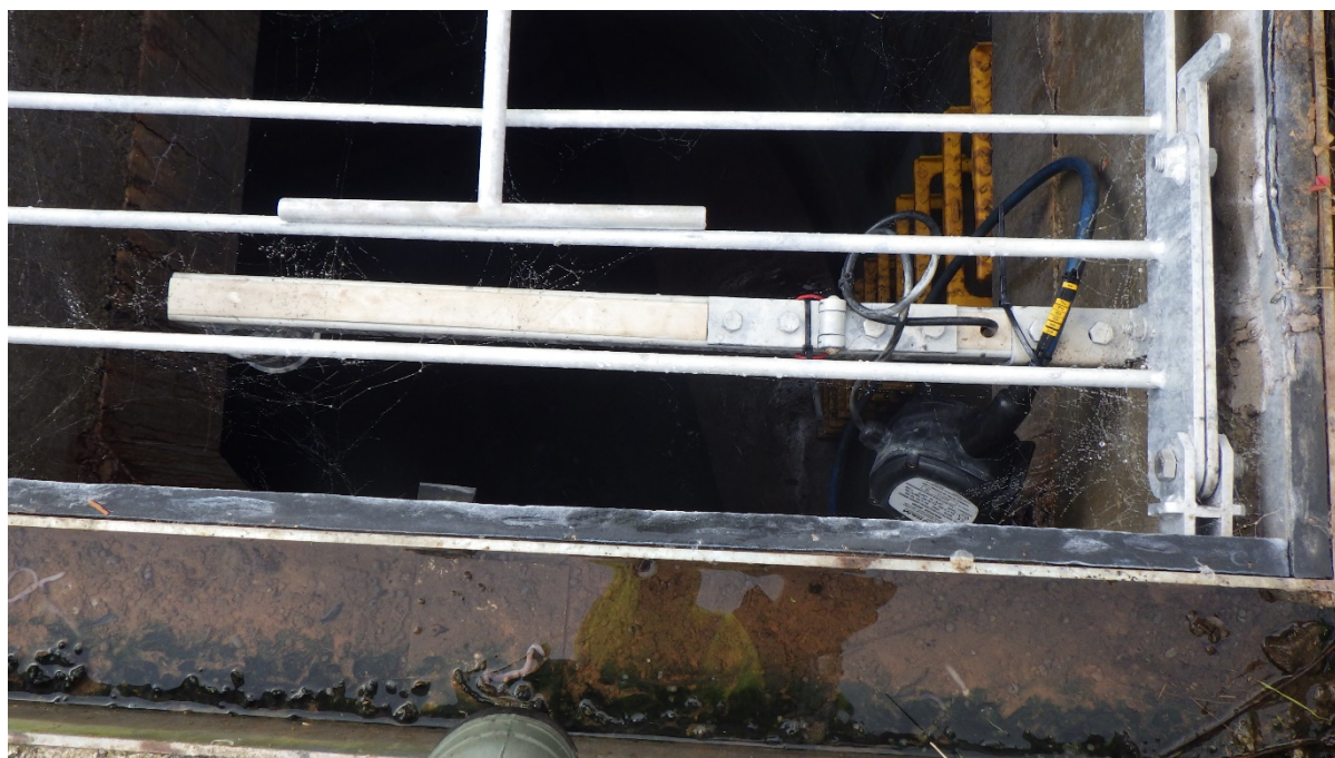
Figure 9: Site visit photo – Telemetry equipment is located in this chamber at ST2392281377.
