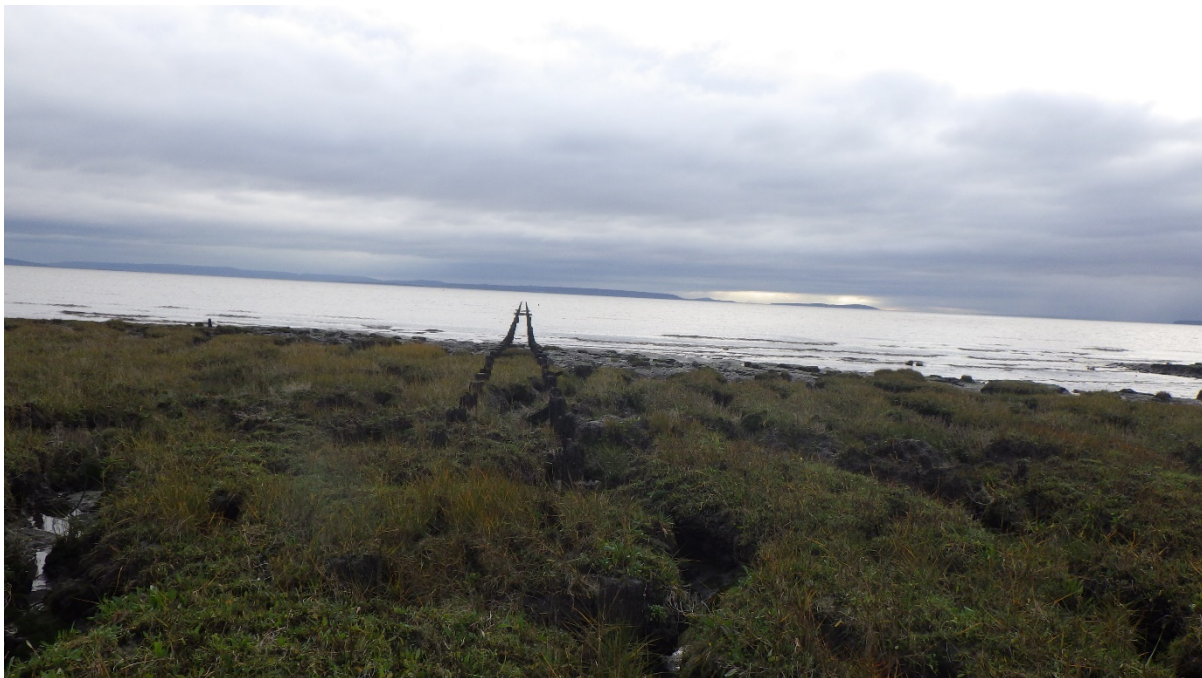
Figure 10: Site visit photo – Storm outfall submerged and inaccessible at the time of the visit.
