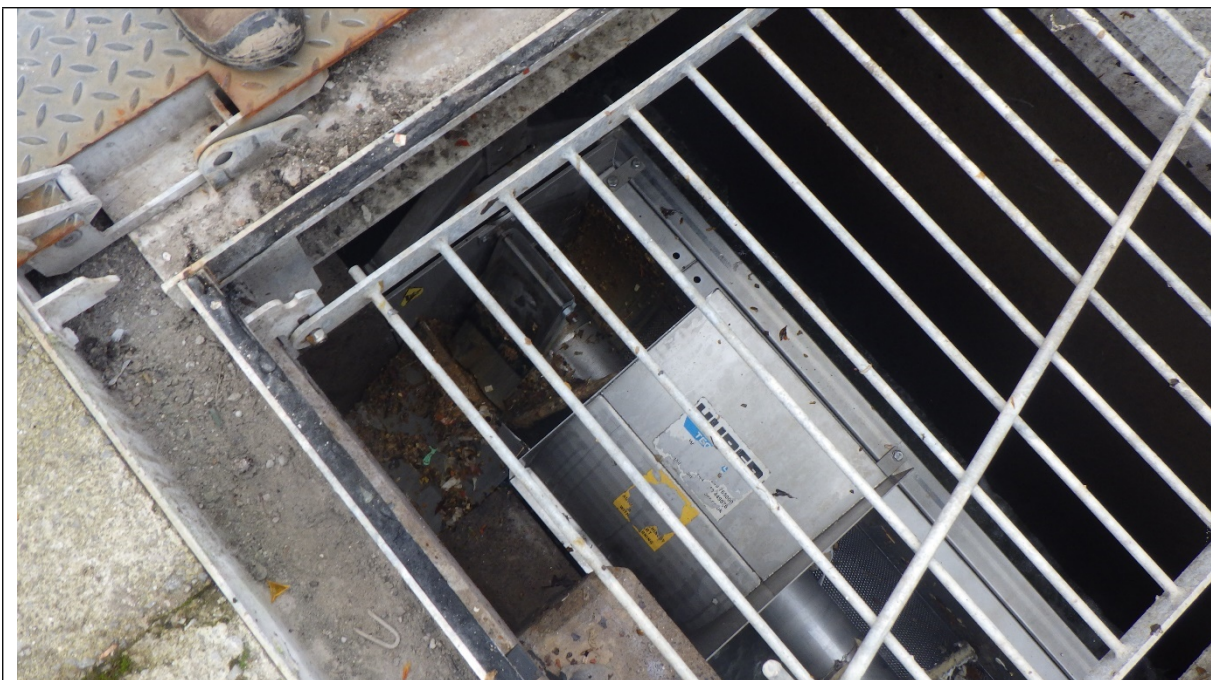
Figure 1: Site visit photo – flipper arms clearing the screen of debris. This debris is then returned to foul for treatment and not discharged.
