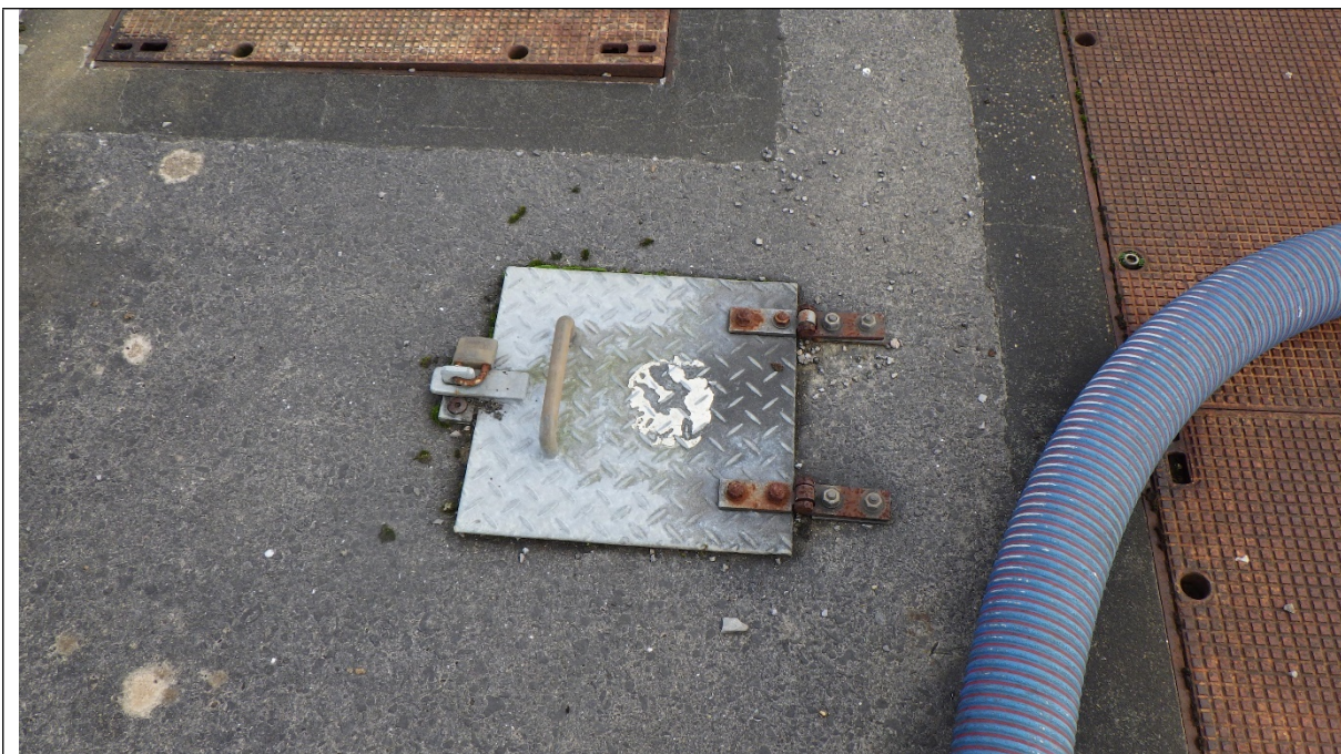
Figure 8: Site visit photo - Clearly accessible sample point
