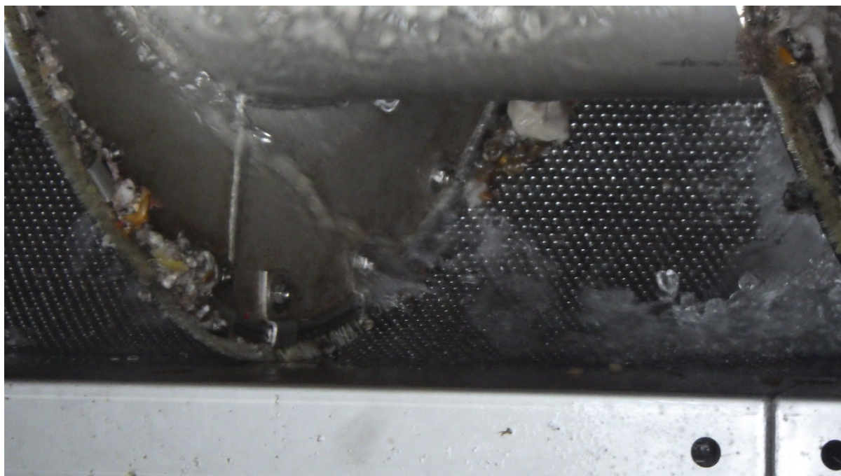
Figure 4: Site visit photo – The screen in good working condition at the time of the visit.
