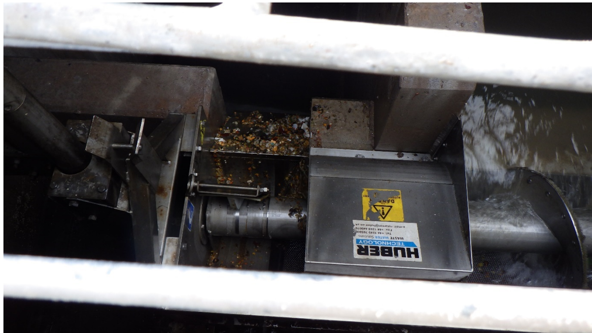
Figure 2: Site visit photo – Screening process where flipper arm can be seen removing larger debris for return to treatment.
