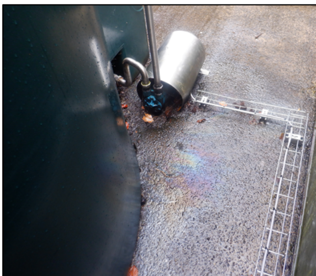
Image 6 (a) – showing an oil sheen on the flooring around the oil storage vessel, taken at 11:14 on 19 October 2023
