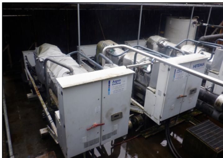
Image 4 – showing chiller compressors fully covered with lagging insulation, taken at 11:20 on 19 October 2023
