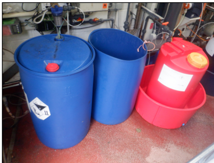
Image 7 (b) – showing container holding sodium hypochlorite present within the boiler room without secondary containment, taken at 12:11 on 19 October 2023
