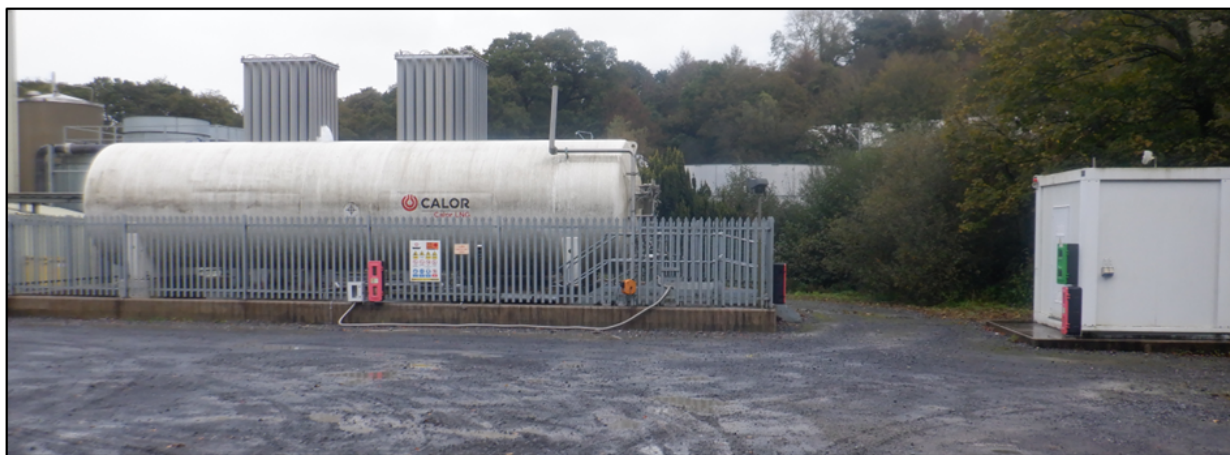
Image 3 – showing LNG compound and telemetry station located at the rear of the site, taken at 11:09 on 19 October 2023
