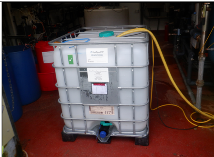
Image 7 (a) – showing IBC holding refrigerant antifreeze stored within the boiler room without secondary containment, taken at 12:10 on 19 October 2023
