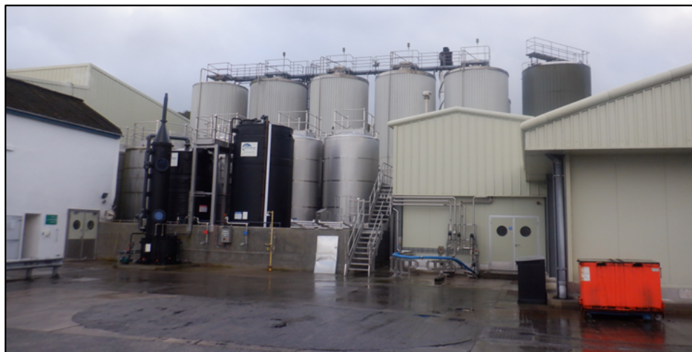
Image 1 - showing CIP system located in front of the milk silo vessels with acid scrubber system, taken at 10:34 on 19 October 2023
