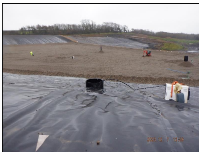
Figure 1 - Unsealed Leachate Sump (Cell 13)
