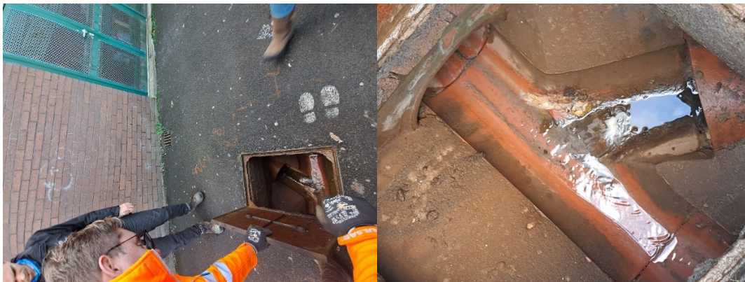
Figure 2. Evidence of ragging in the surface water system outside of the plant room where the discharge gully enters the system.
