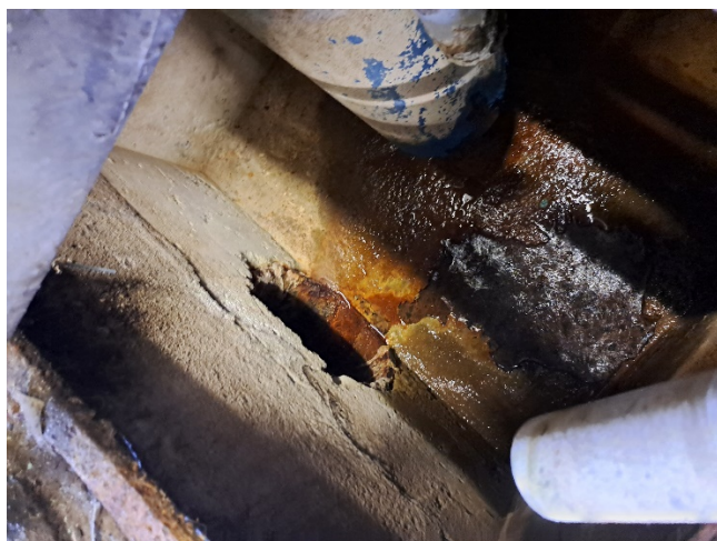
Figure 1. Discharge point/ gully including the trickle discoloured discharge from the white PVC pipe from the heaters (foreground).
