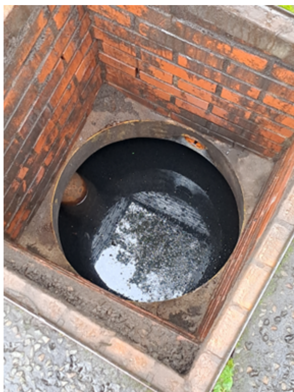
Figure 4. Contents of the tertiary interceptor chamber.
