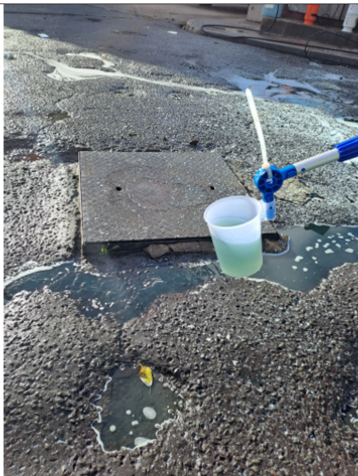
Figure 8. Blue liquid present within the soakaway system.
