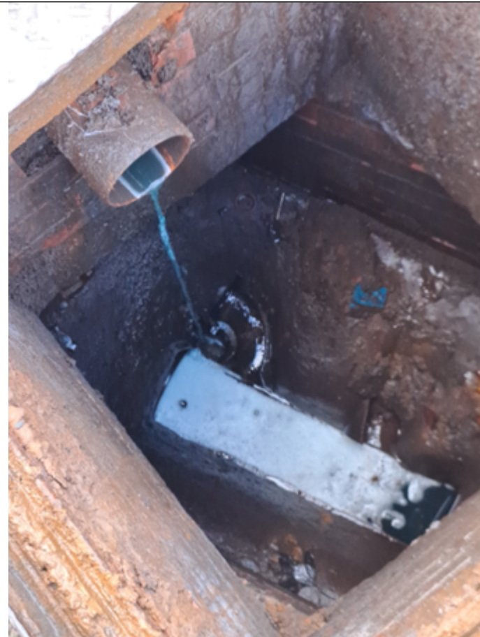
Figure 6. Evidence of blue water contaminated with detergent and soap suds coming from the carwash entering the soakaway system inlet.
