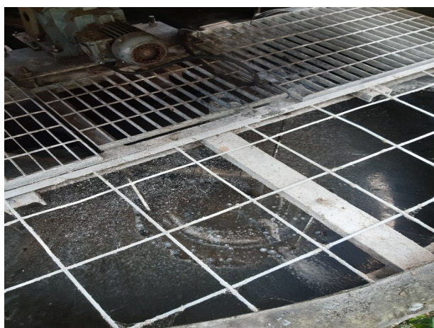
Figure 3: Final chamber showing aeration of effluent
