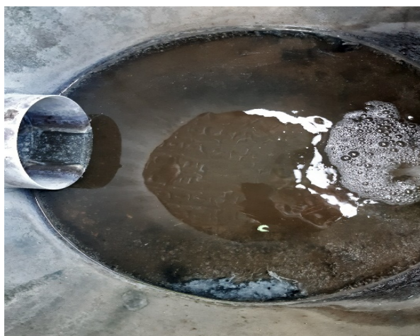
Figure 5: Inspection chamber showing staining and some scum
