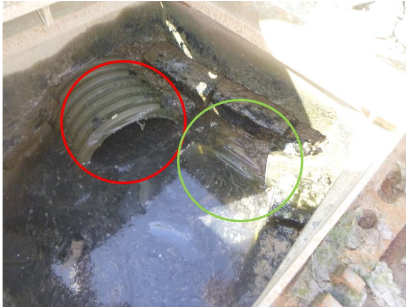
Photograph 5: Surface water (red) and final effluent (green) chamber
