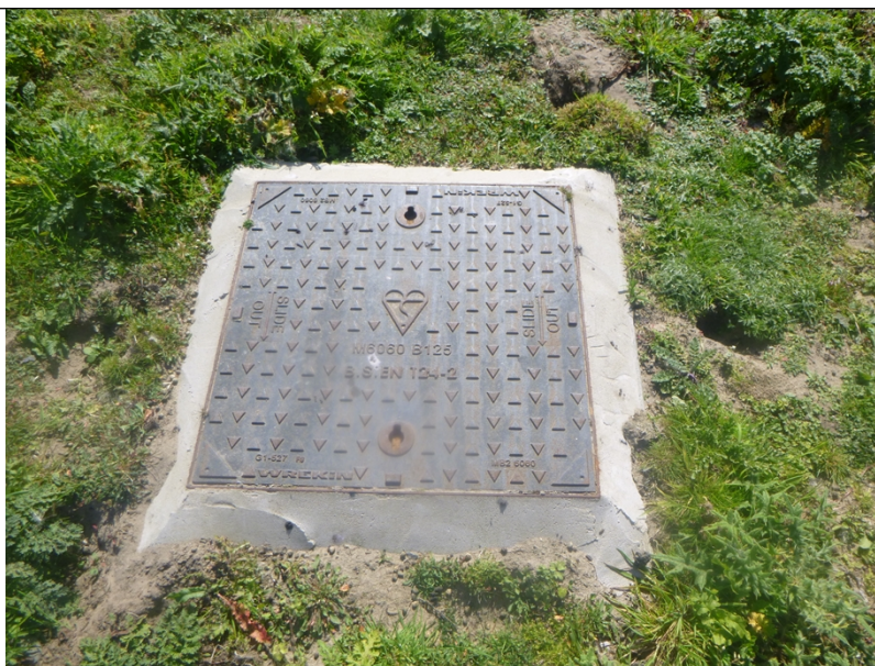
Photograph 3: Final effluent sample point
