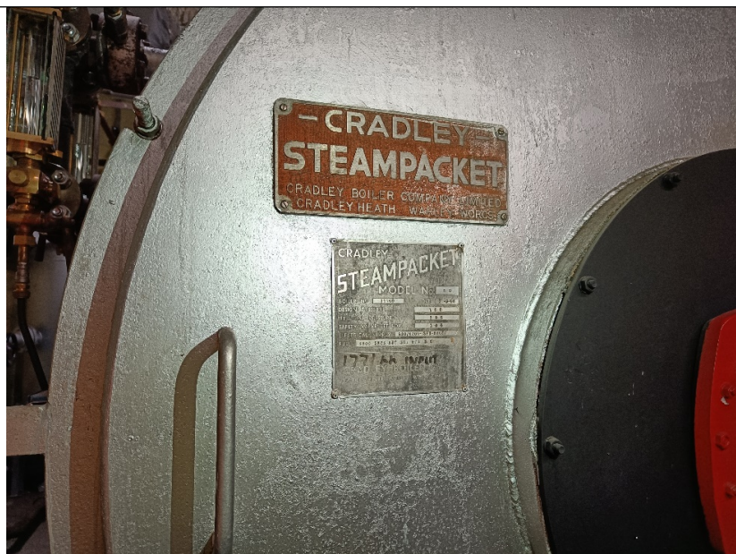
Photo – boiler with 1771kW input written on the plate.
