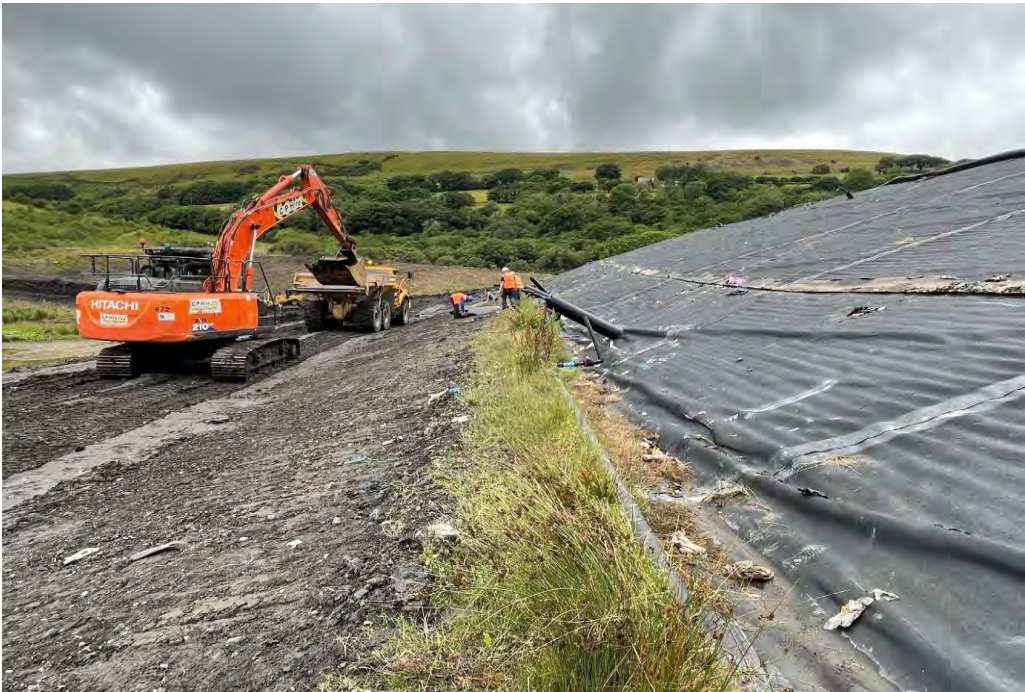
Rain Flap Removed
