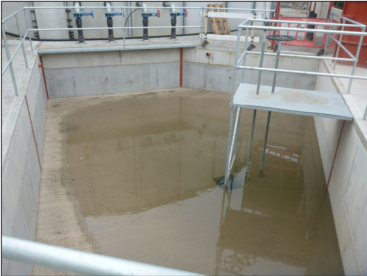
Figure 6. Photograph showing (W1) clean surface water sump and double valves for outlet.
