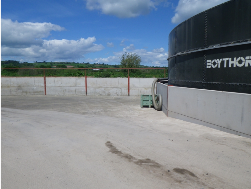
Photo 3: Drain and pumping equipment
