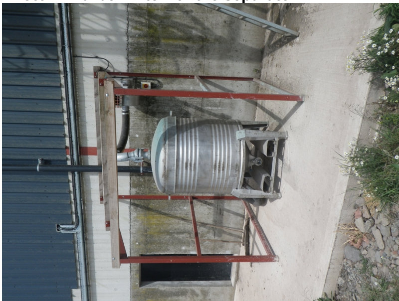
Photo 2: Carbon filter for the separator
