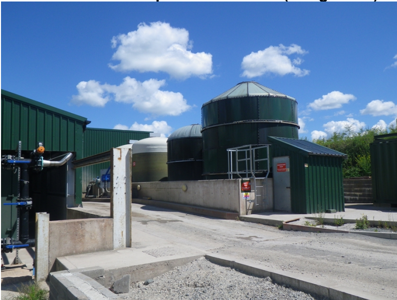
Photo 6: Two new liquid waste tanks (foreground) in bunded area
