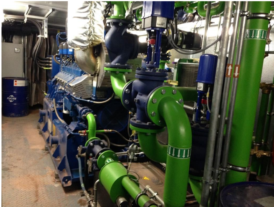
Figure 3.8: Existing CHP Plant
