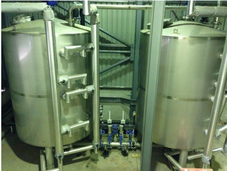
Figure 3.5: Existing Pasteurisation Tanks
