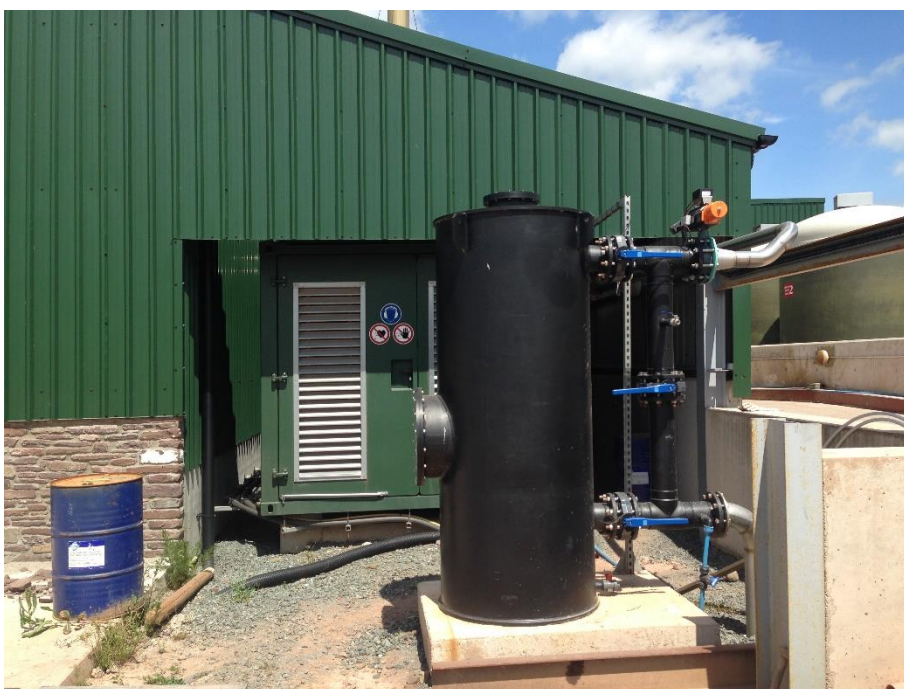
Figure 3.7: Existing Dry Carbon Filter Unit
