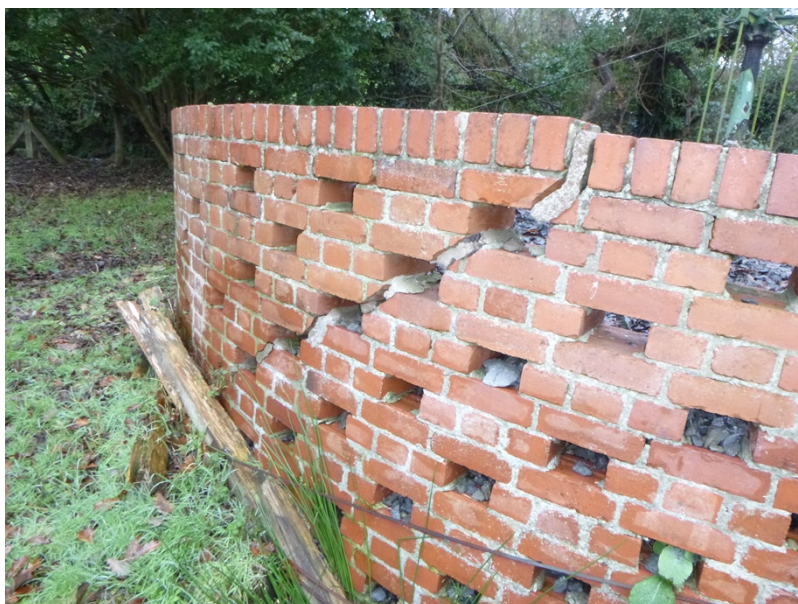
Photograph 5: Crack patched up with cement in filter bed wall
