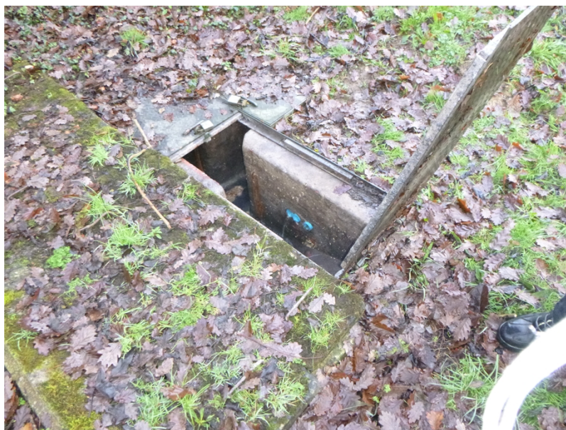
Photograph 1: Capel Bangor WwTW inlet. Surface water/land drainage pipes in blue.
