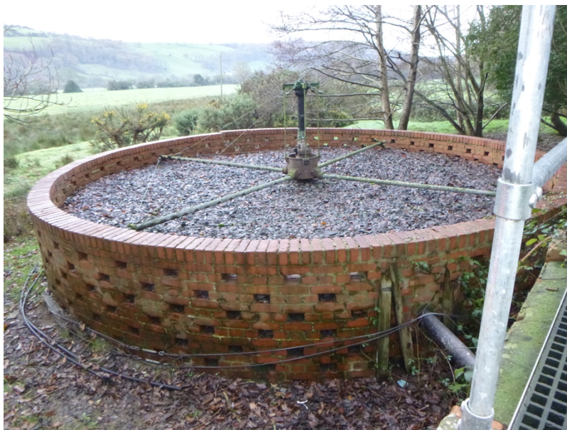
Photograph 4: Stone media filter bed at Capel Bangor WwTW and distribution chamber (foreground right)
