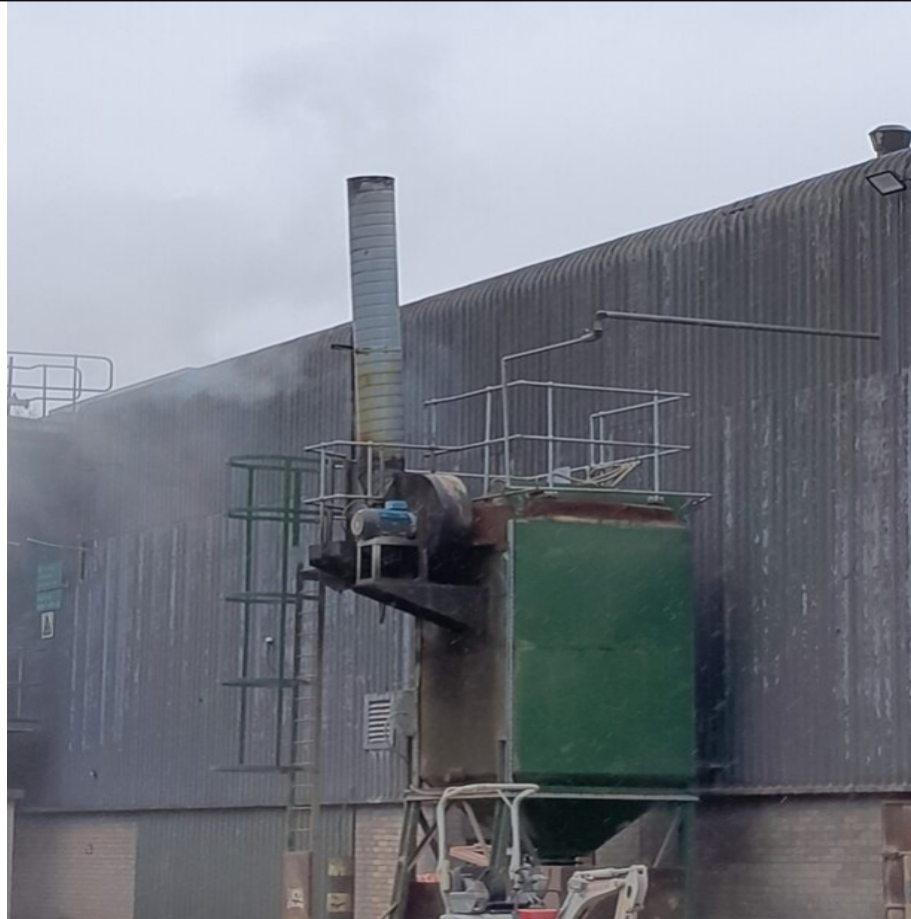
Photo 1 - showing vapour emanating from the dryer
