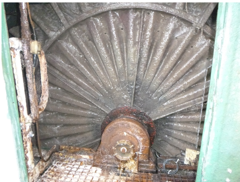
Photograph 5: Rotating biodisc at Rhydyfelin WwTW
