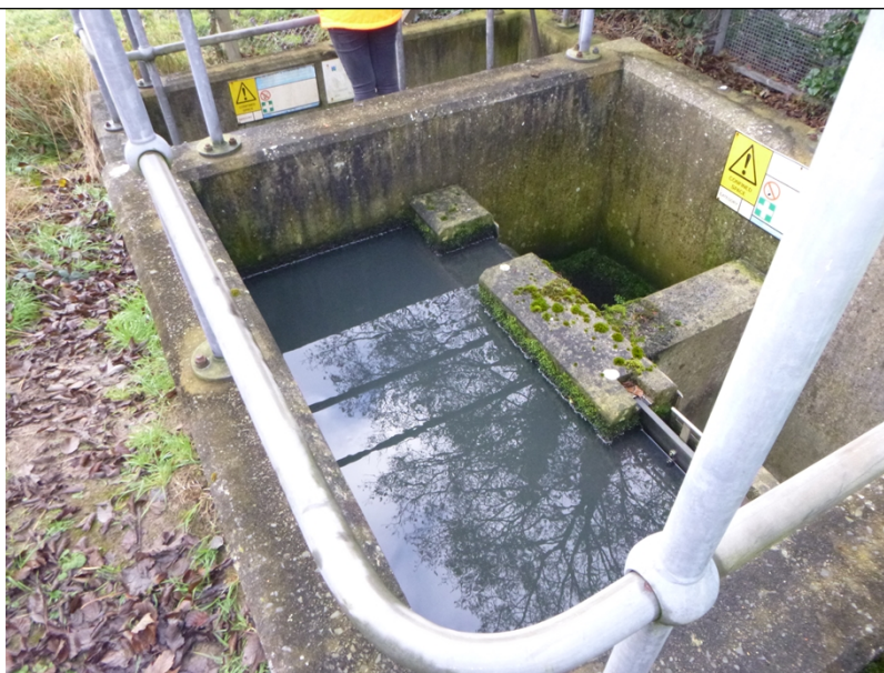
Photograph 6: Final settlement tank
