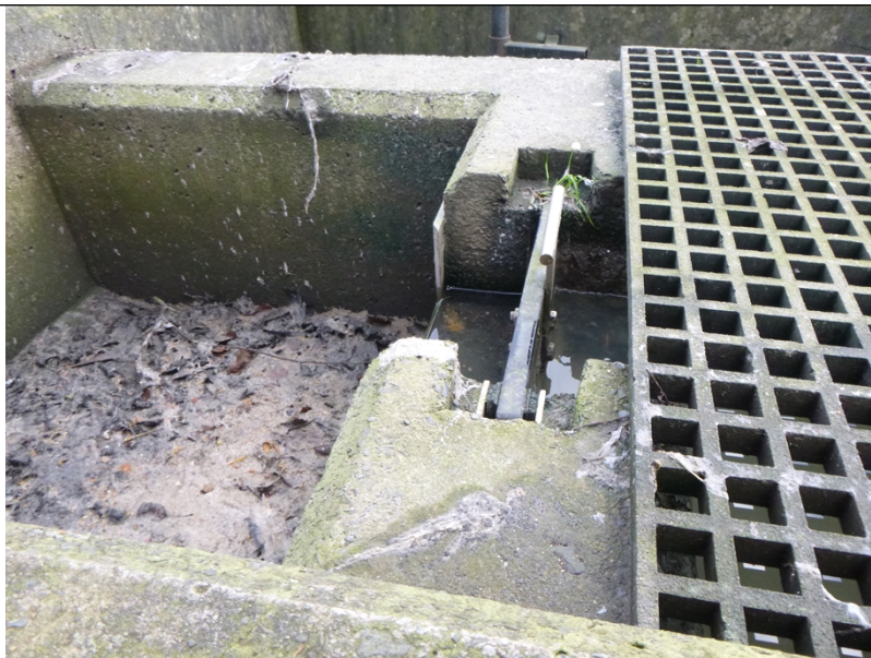
Photograph 4: Overflow at inlet
