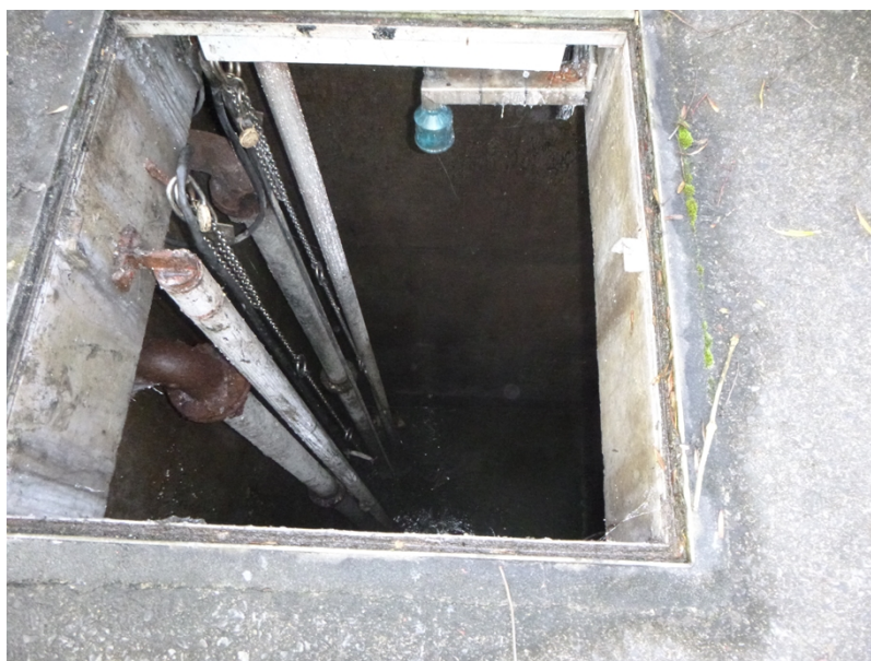
Photograph 1: Pumping station foul well
