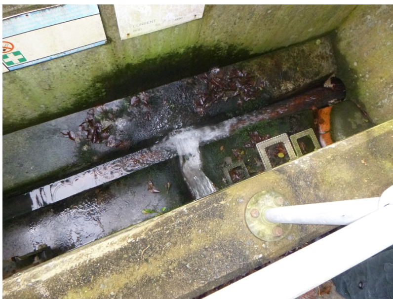
Photograph 7: Final effluent sampling point
