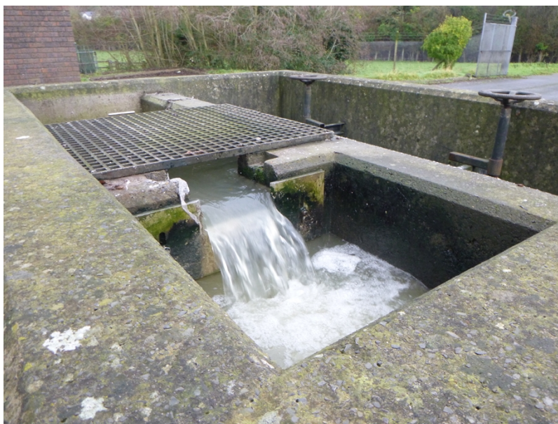
Photograph 3: Rhydyfelin WwTW inlet
