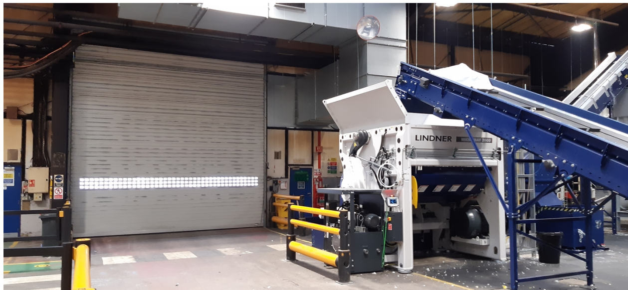
Photo 7 - Air Handling Unit (AHU) installed to mitigate excess noise emissions
