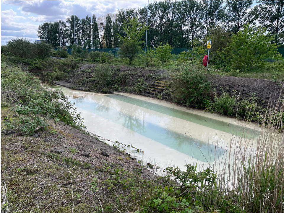
Plate 7-1 Surface water above concrete plinth (May 2023)
