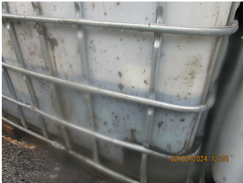
photo 5 liquid pooling at the bottom of the battery container
