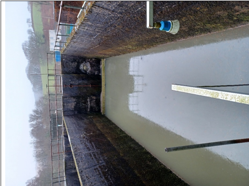
Image 3: One of 3 storm tanks at holding capacity
