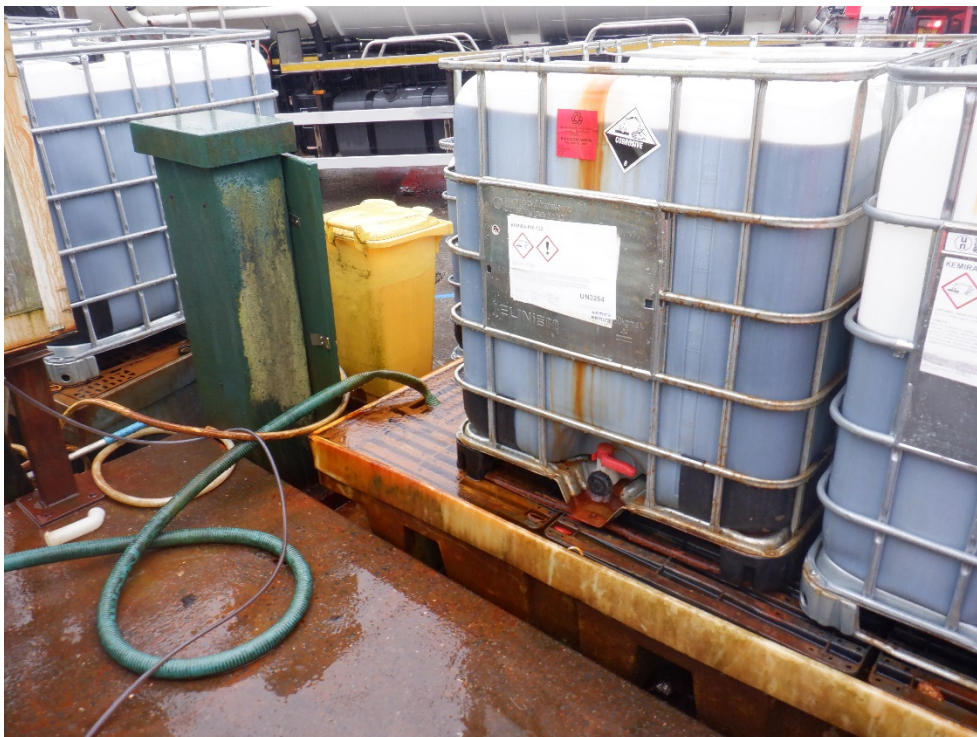
Figure 7 IBC's of Ferric Chloride stored on overtopping bunds
