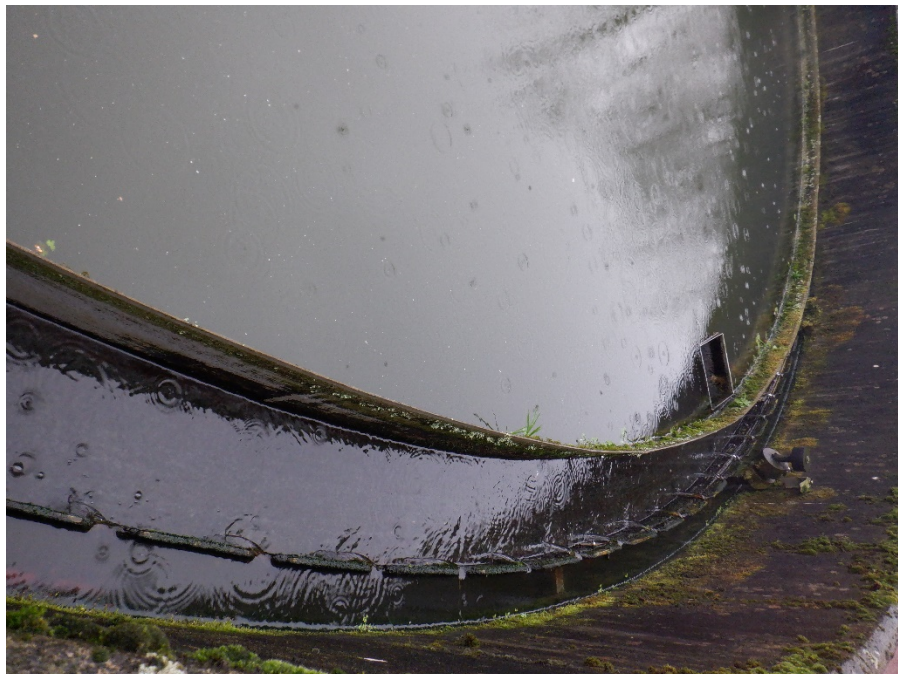
Figure 6 Final effluent from the final settlement tanks
