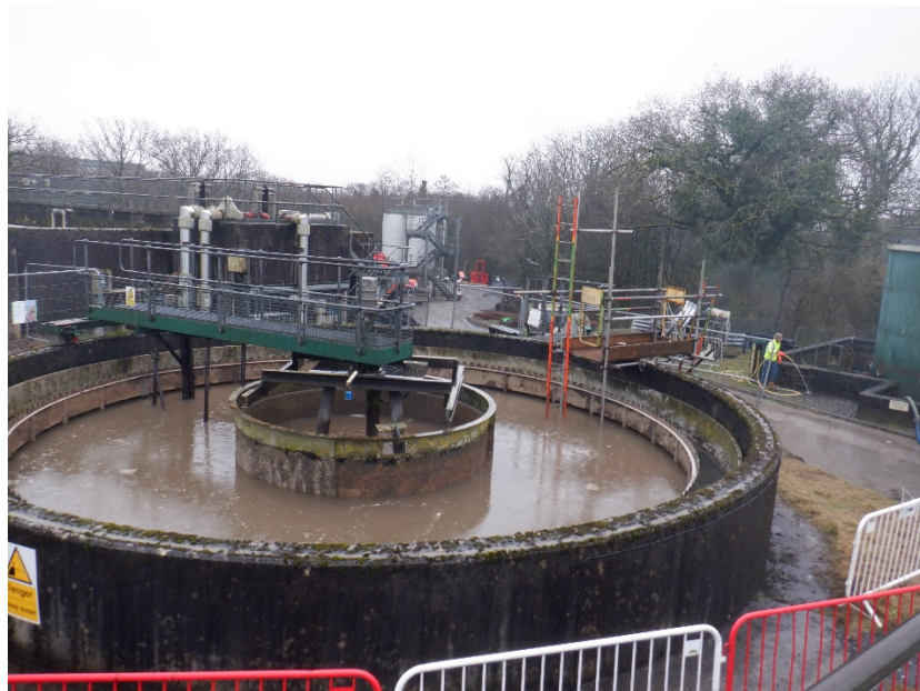
Figure 2: Old Primary Settlement tank acting as storm storage.
