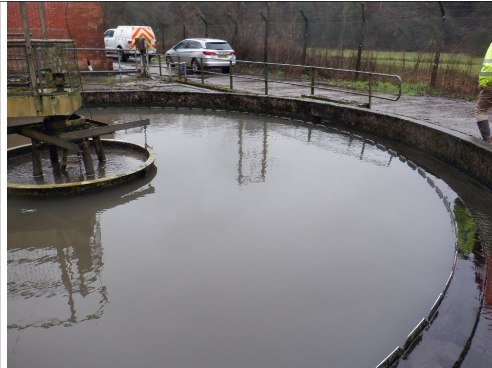
Figure 5: Final Settlement tank
