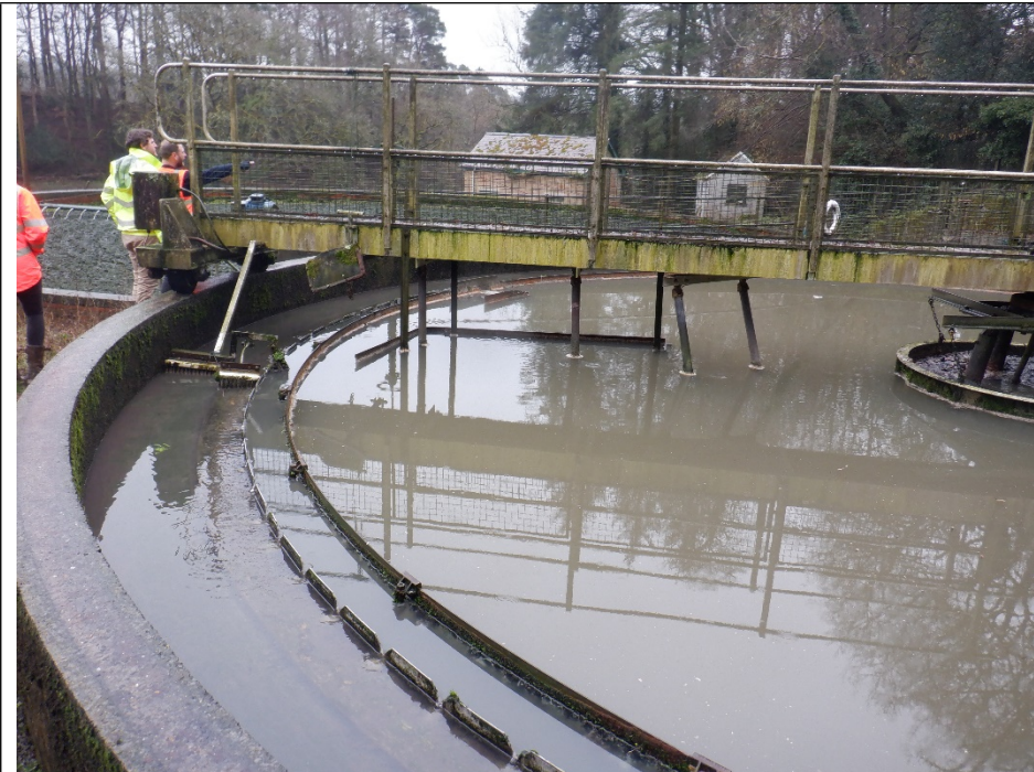
Figure 4 Primary settlement tank
