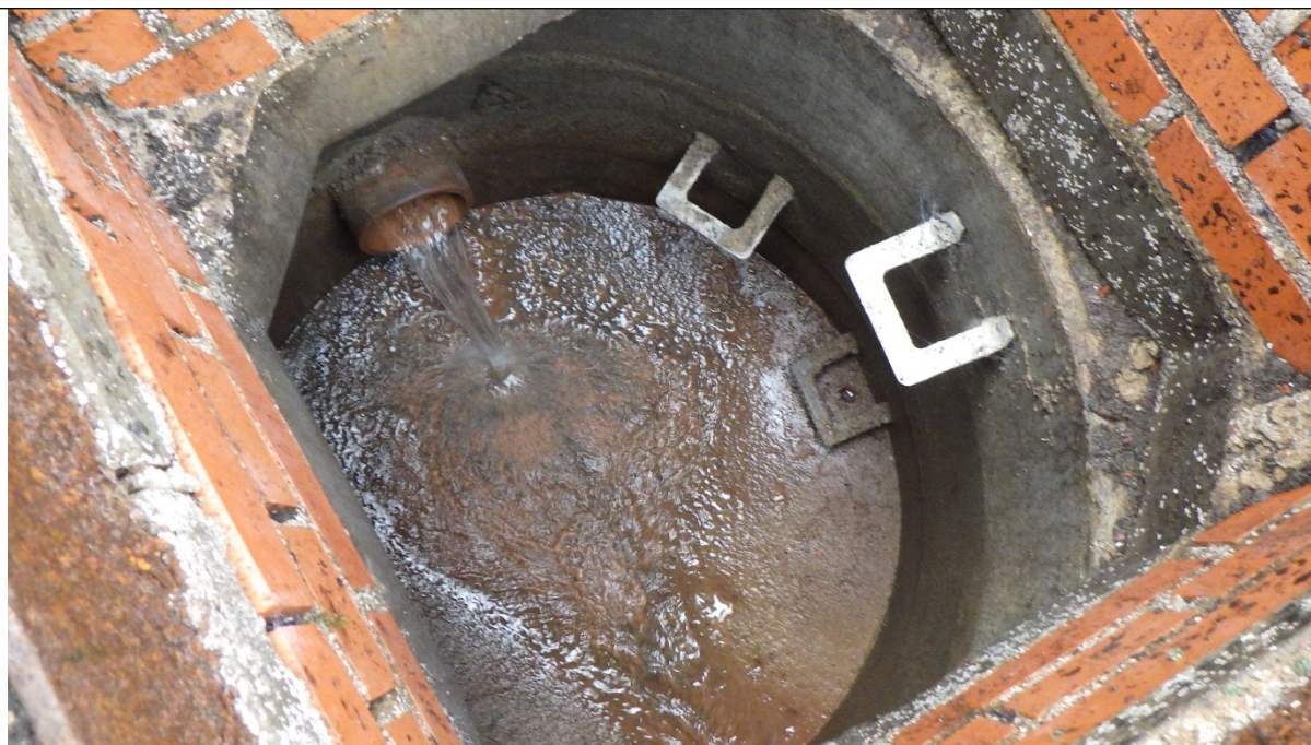
Figure 7 – Site visit photo: The treated effluent as it is discharged from the filtration unit. Flow rates appear higher than the consented levels.
