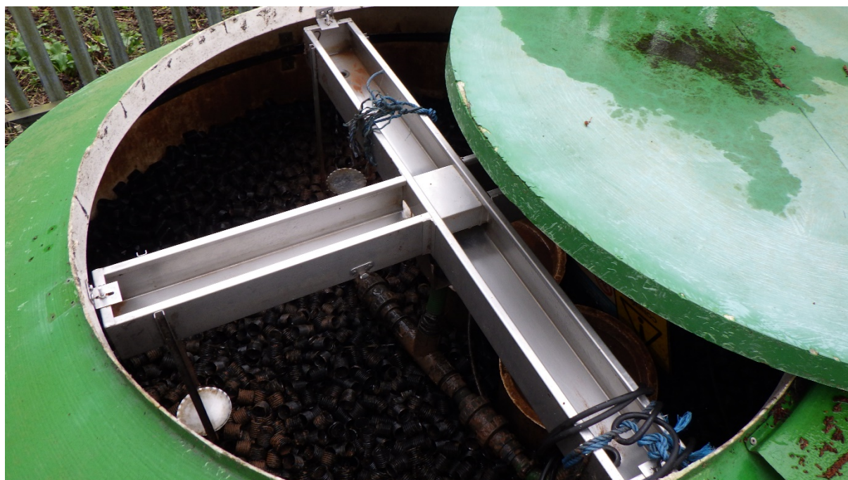
Figure 5 – Site visit photo: The filtration unit in operation at the time of the visit.
