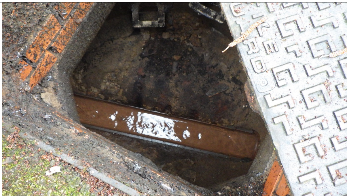
Figure 4 – Site visit photo: The effluent as it flows from the solids separation chamber to the filtration unit. Effluent is clear of all solid waste and has a moderate flow.
