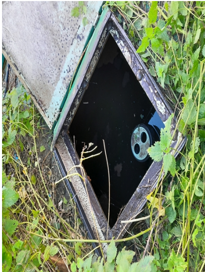
Sample Point Chamber (Photo 4)
