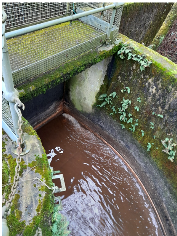
Image 1 – Bypass Channel Leak
