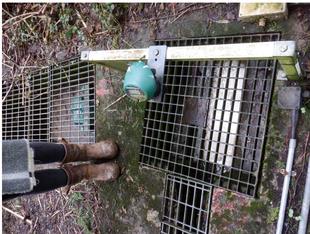
Figure 1: Inlet to the works with the storm overflow in the background.
