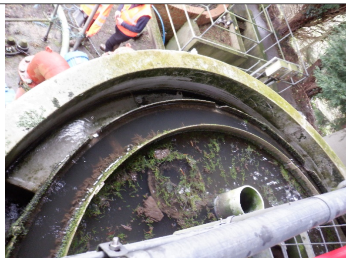
Figure 4: Final settlement tank
