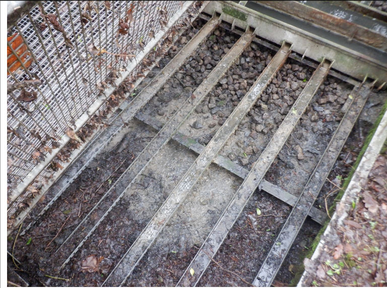
Photo showing build up of solids on filter bed.
