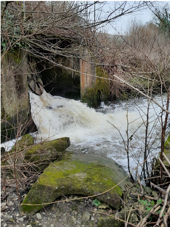
Image 2 – Discharge Point for Settled Storm Sewage
