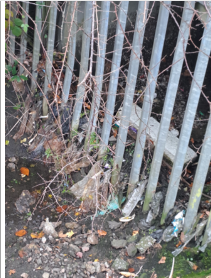
Figure 2. Evidence of detritus and litter causing a partial blockage of the culvert exit.
