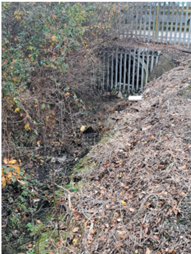
Figure 1. Location of culvert exit into gully which feeds into the River Rhymney.
