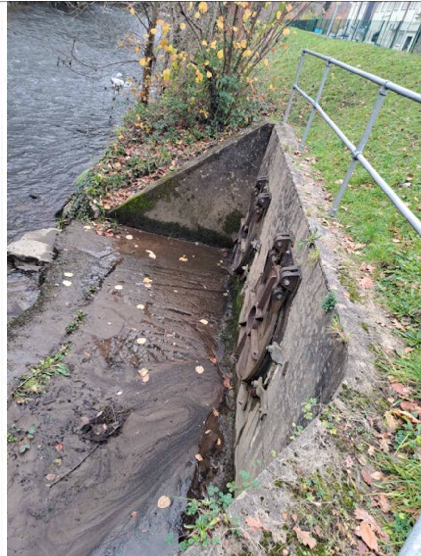
Figure 3. Discharge point into the River Rhymney, with silt present on the bottom of the outfall.
