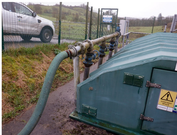
Figure 1: An image of pipes used for desludging.
