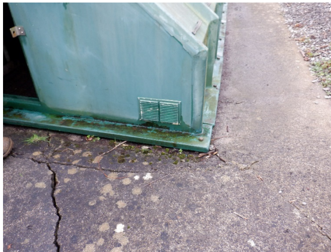
Figure 3: An image of the concrete base the RBC tank is built upon..
