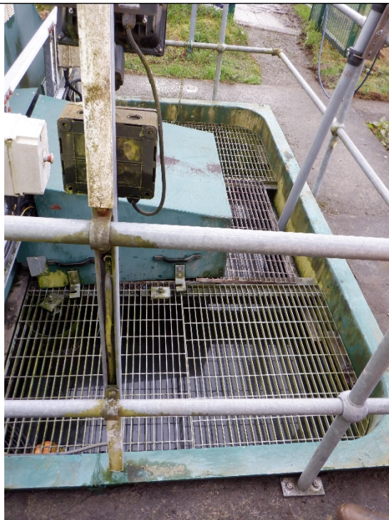
Figure 4: An image of the final settlement tank following on from RBC treatment.
