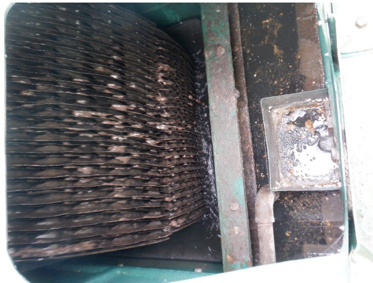
Figure 2: An image of a RBC facilitating secondary treatment of effluent. The channel in front of the RBC is used for primary settlement.
