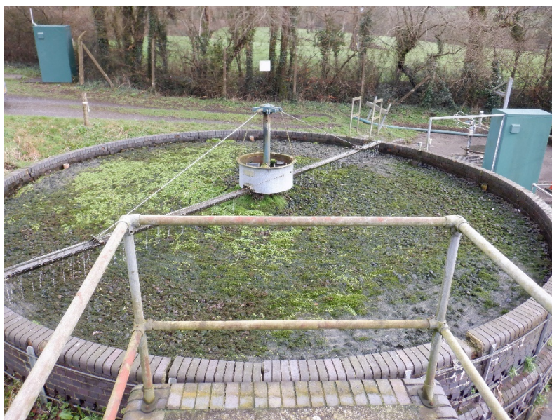
Figure 3: An image of the percolating filter bed.
