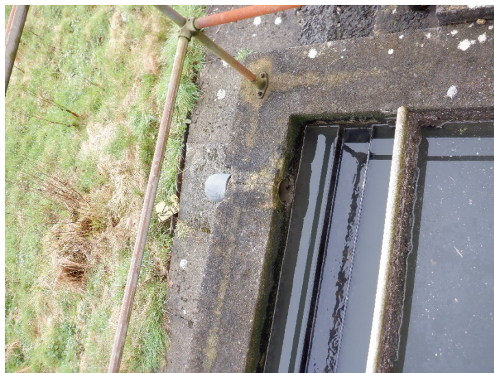
Figure 2: An image of an overflow pipe situated in the PST.
