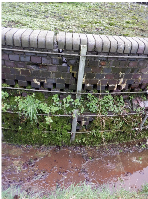
Figure 4: An image showing a crack in the brickwork of the percolating filter bed.
