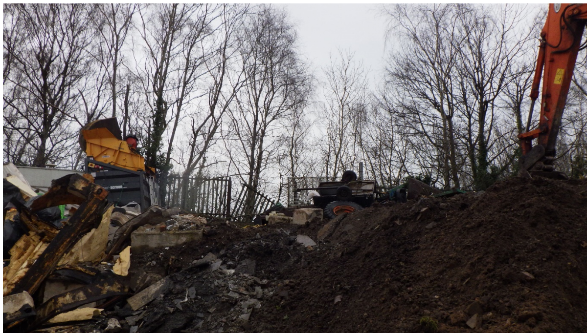
Damaged fence on site
