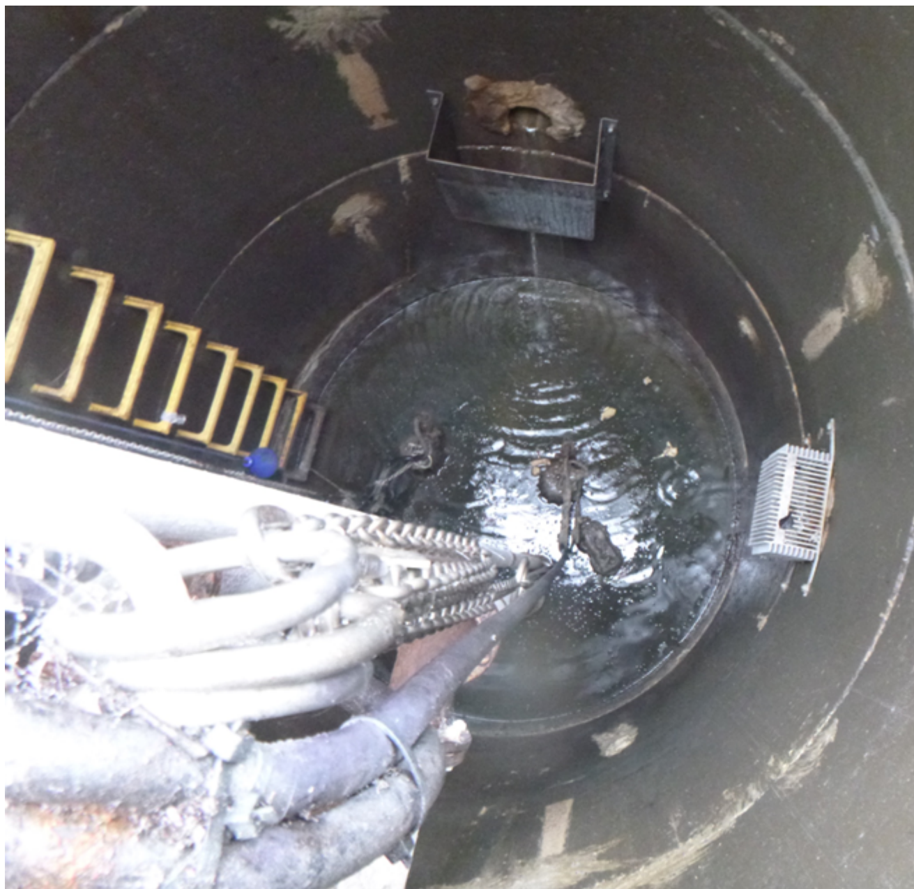
Figure 1: Tank at Erw'r Brenhindedd Pumping Station.
