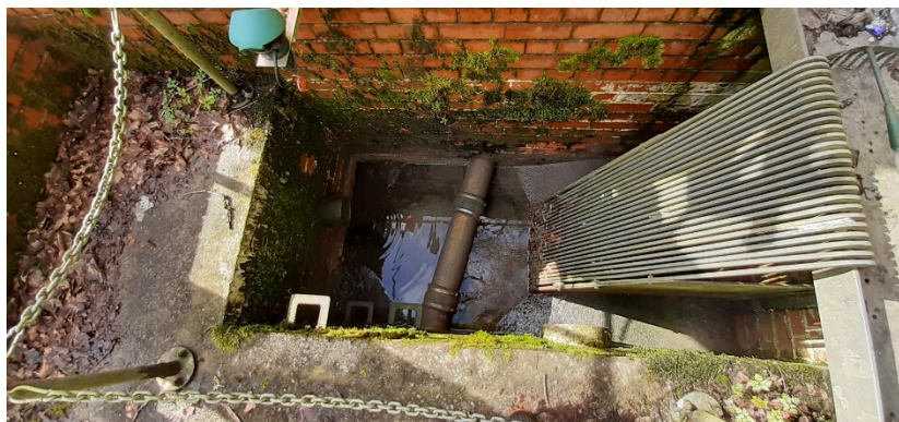
Figure 2: An image showing the chamber where final bar screening of storm effluent takes place before being discharged to the receiving watercourse.
