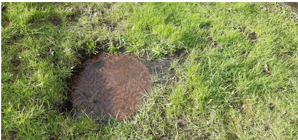
Figure 5: An image of a manhole at the site with leaking rainwater.
