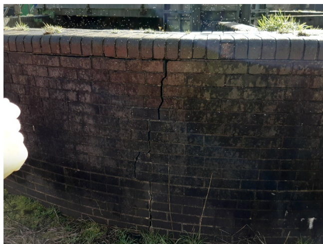
Figure 3: An image of a crack in the brickwork of the splitting chamber.
