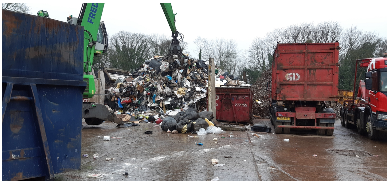
Photo 4 - General wastes stored in designated / segregated bays
