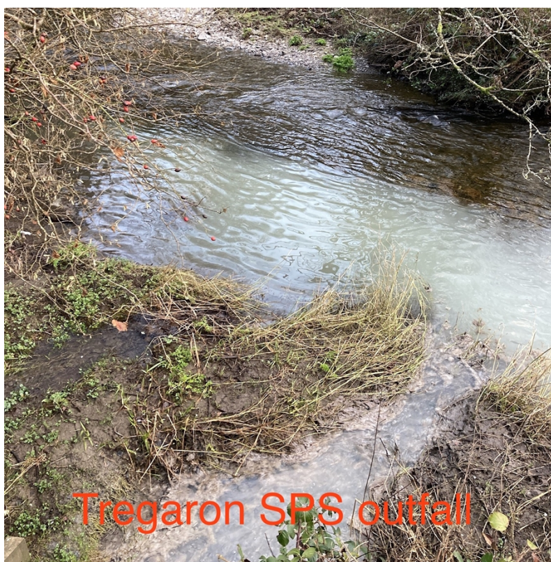
Photograph 4: Grey plume in Afon Breninig at Tregaron SPS outfall on 08 January 2024. Photograph courtesy of DCWW.
